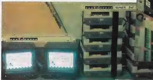
(Above) This is just one of the panels in the control room. There are several more to keep an eye on!
